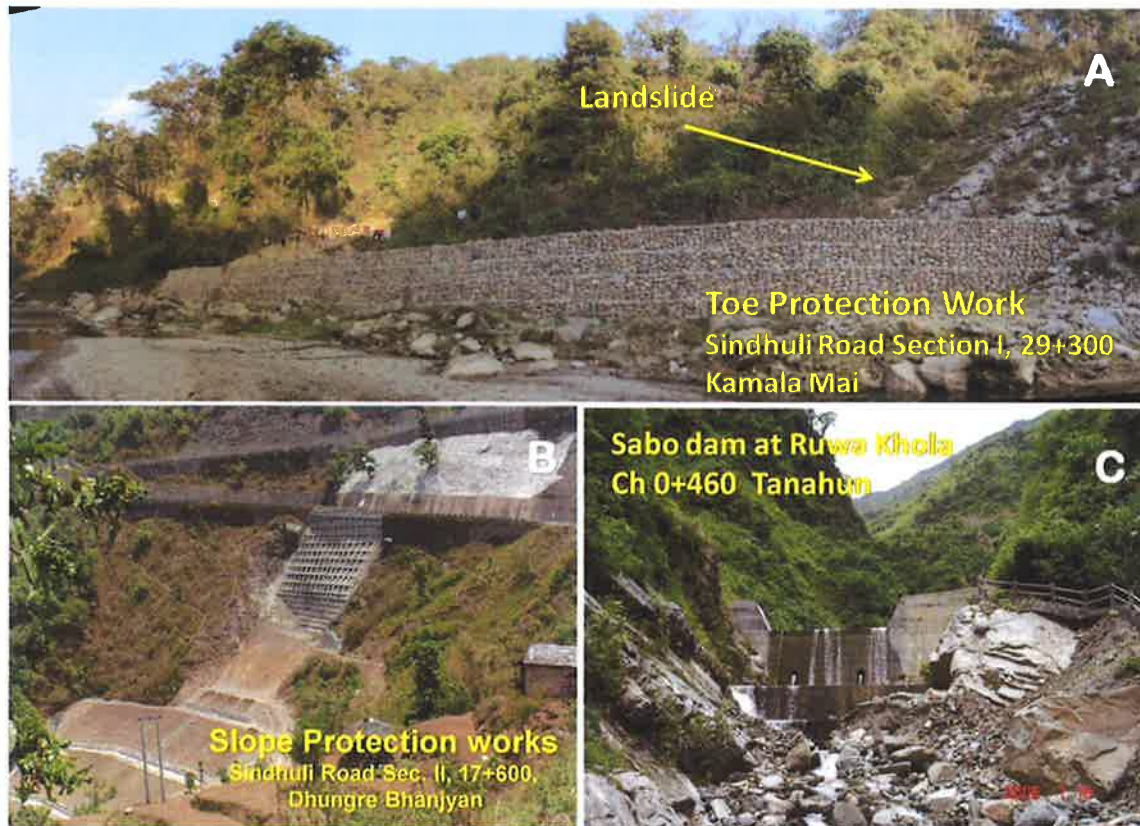
Figure 10. Landslide mitigation measures implemented in Nepal. A) Toe protection works to mitigate slow moving landslide, Sindhuli Road, Section I, 29+300m (Amatya & Mori, 2018), B) Slope protection works by anchoring to mitigate slope failure, Sindhuli Road, Section II, 17+600, (Amatya, 2016), C) Debris flow mitigation works by Sabo dam, Ruwa Khola, Marshyangdi Hydropower, 0+460, Tanahun (Pandit, 2009).
